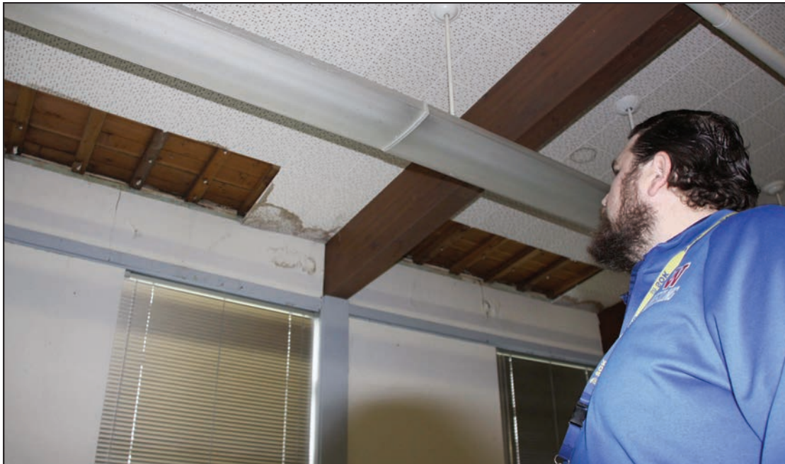
Seven Oak Principal Colin McHill surveys water damage to a classroom ceiling from roof leakage at the nearly 70-year-old school. - Photo by Scott Swanson
