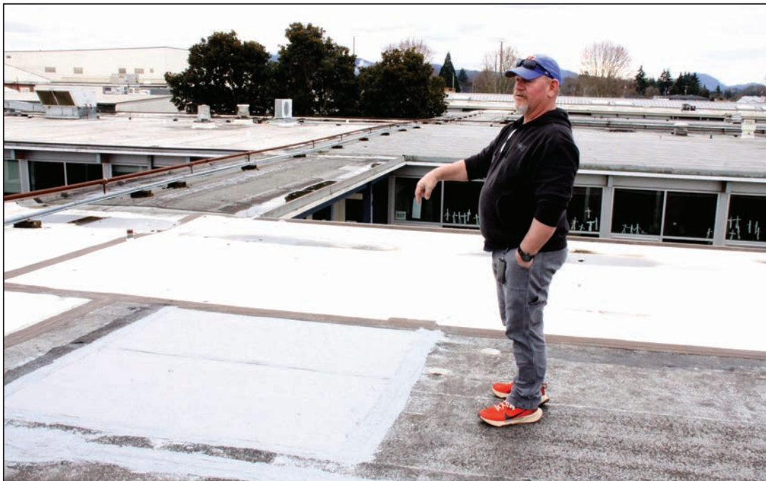
Brian Eilers talks about repairs that have been made to the Lebanon High School roof over one of the original classroom wings. The original asphalt rolled roofing was coated with white mineral granule surfacing that has largely disappeared over some 70 years, requiring patching and other repairs visible as lighter sections and reducing the roof's ability to reflect sunlight during the summer.
