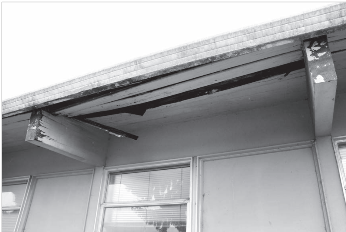
Damage to the soffit of an eave on one of the original classroom wings at Seven Oak Middle School indicates leakage. The overhang has already been cut in by approximately a foot due to rotting of the beams.
