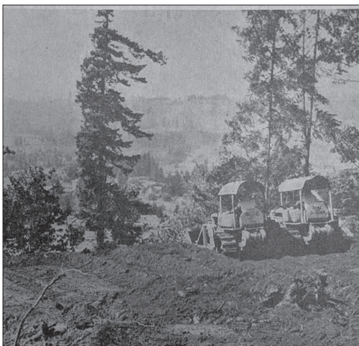
Two "Cat" operators level off the hill above Sweet Home for the city's new 750,000-gallon water reservoir in 1951. The city water superintendent announced this week one reason there is a water shortage is due to limited storage capacity.
