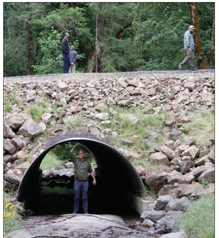
Scott Bruslind, SSWC president, gauges the height of a newly installed culvert on the South Santiam 500 Line.
