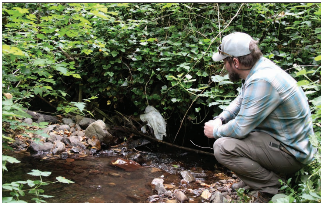
Tyrell Styhl inspects a culvert on Mouse Creek that is overgrown, undersized, and subject to clogging by trash and debris. A planned replacement is in the works. — Photo by Scott Swanson
