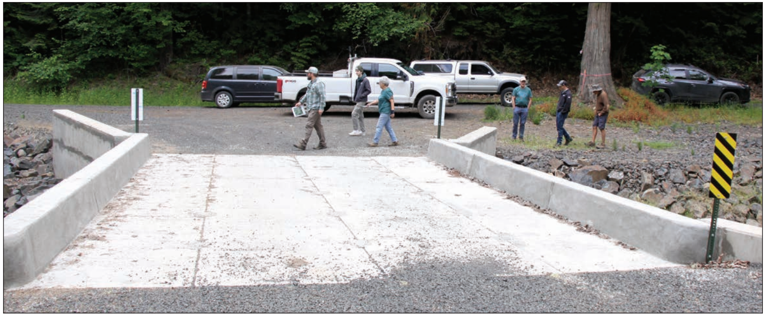
Tyrell Styhl, executive director of the South Santiam Watershed Council, center, leads a tour focusing on improvement projects, such as this new bridge on the Ames Creek 400 Line. – Photos by Scott Swanson
