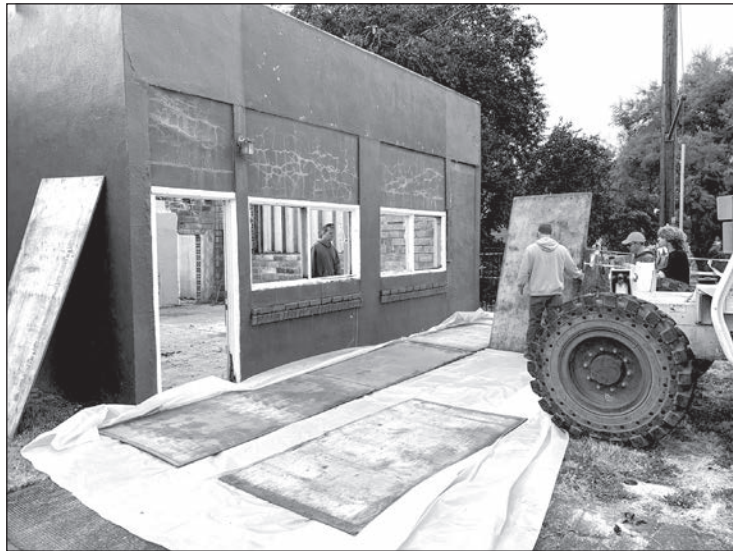
Workers make final preparations before tearing down the front wall of Victorian Chocolate Company. – Kelly Reetz photo
